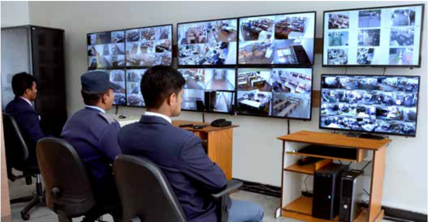
Camera Surveillance Room in the Palada Campus
