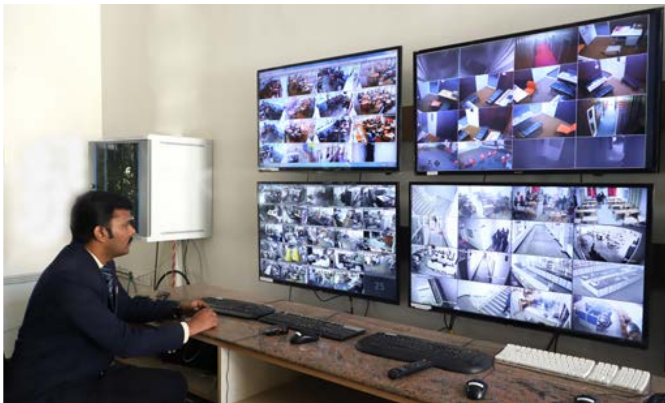
Surveillance room: Monitoring modern CCTV security cameras
